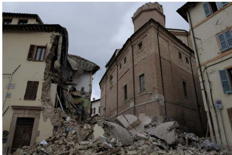
Figure 12 | Camerino (MC) after the earthquakes on 26 October and 30 October 2016. Source: Wikimedia commons.
